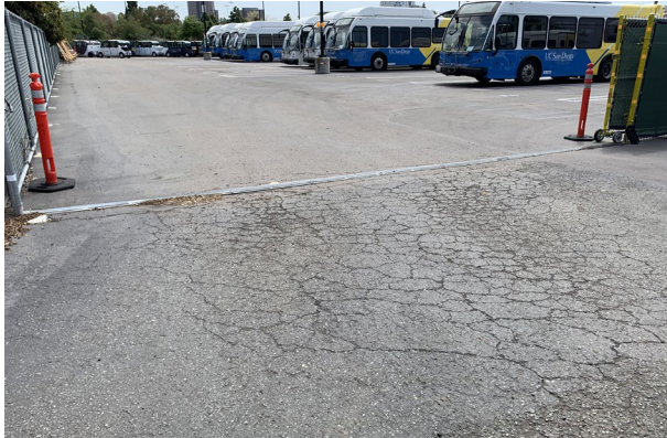
Figure 17: Example of failing pavement conditions at existing facility.
